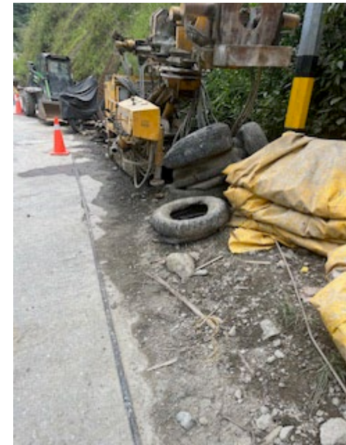
Photo 51: Inadequate waste management
