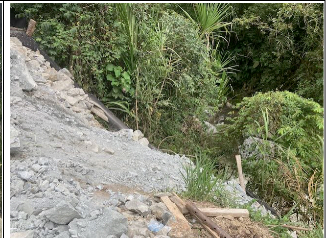
Photo 18: Temporary spoil deposit at upper tunnel portal, at risk of sliding into river
