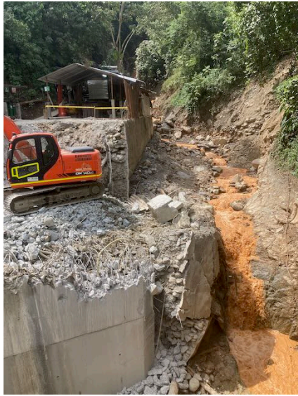
Photo 61: Heavy sediment load of creek at lower tunnel portal, caused by slope failure above, with damaged platform on left
