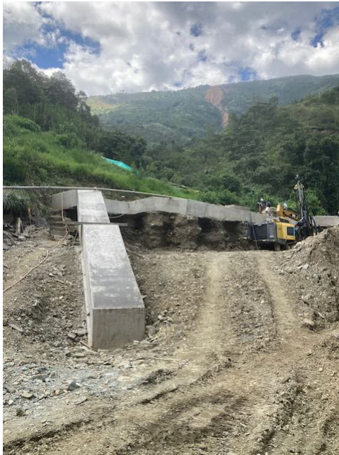
Photo 49: Containment wall between future powerhouse below and spoil deposit from road construction above
