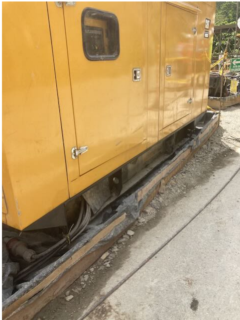
Photo 43: Construction equipment with inadequate containment 2
