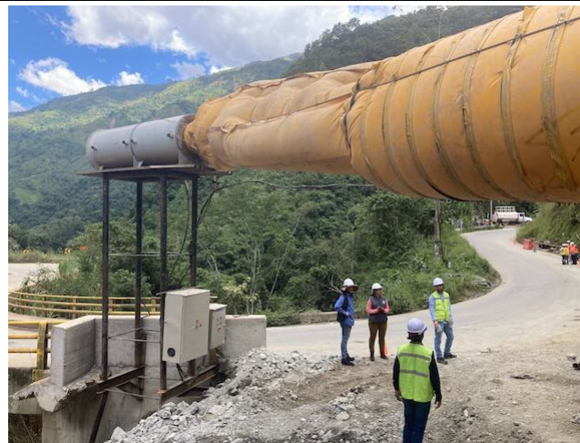
Photo 53: Ventilation at lower tunnel entrance
