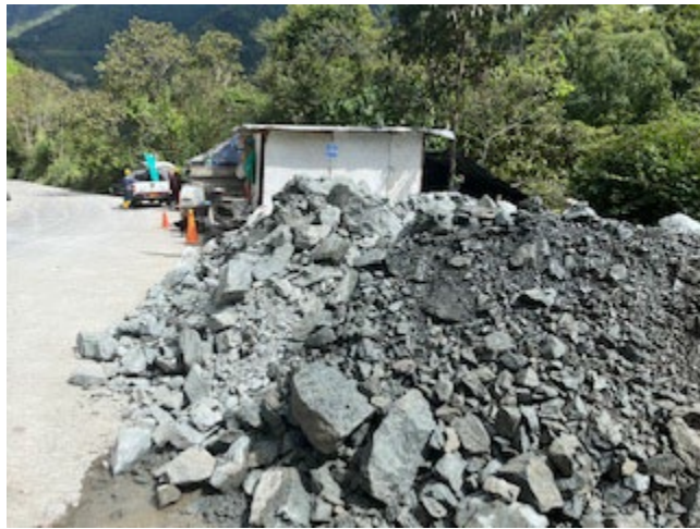
Photo 40: Inadequate containment of excavated material from tunnel
